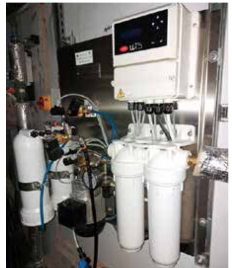
WTS Compact installation (up)
